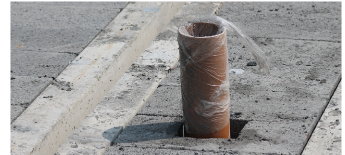
Service Pipe Through Floor
